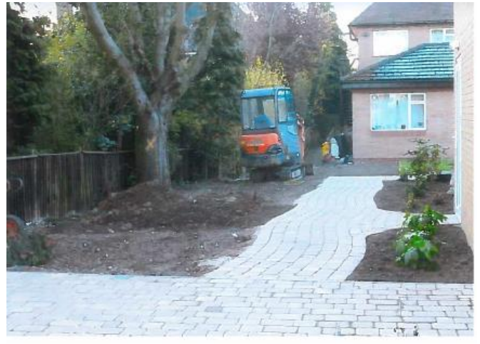
Physical damage and Tree removal
